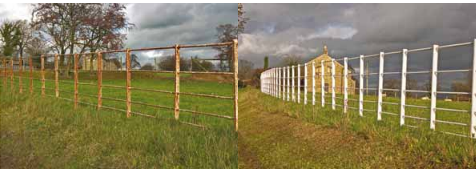
Before and after photos of the railings in Bolton by Bowland which Richard Atton, the local lengthsman, recently completed. What a great difference it makes.
